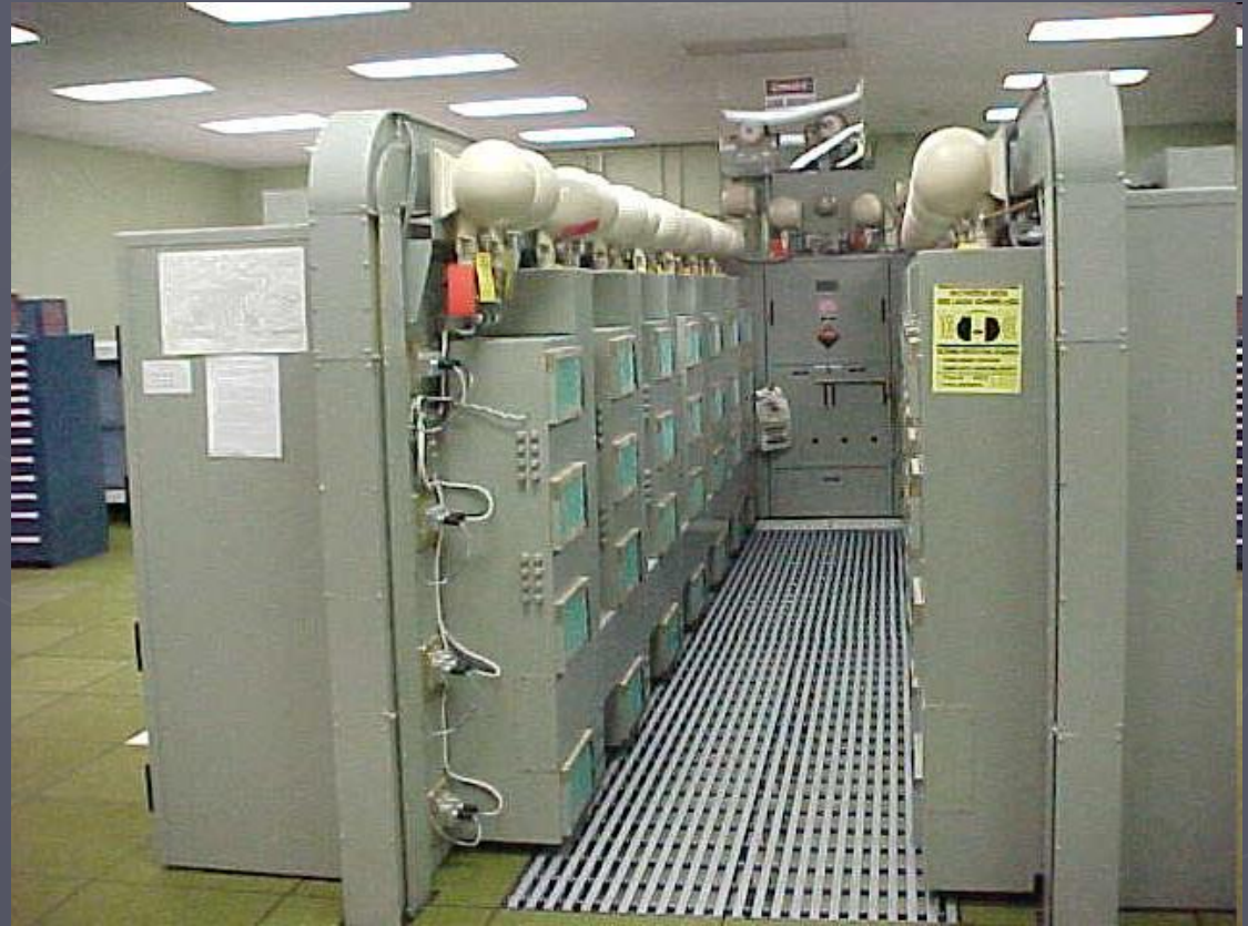
LORAN transmitter bank
